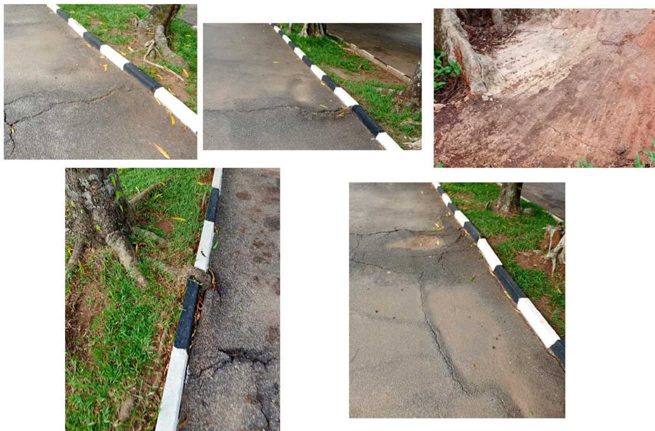
Figure 1: Impact of tree roots on road structures within the survey area
