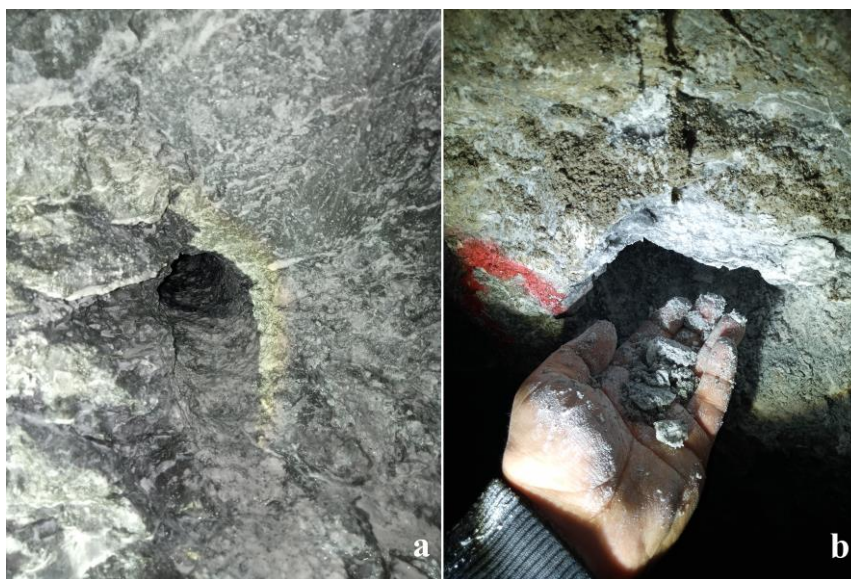
Figure 10. A shown of the dacitic tuff formation: a drill hole (a) and its fragmentation by hand (b)
