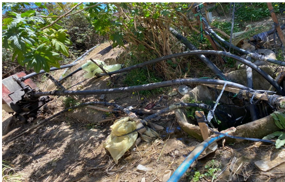
Figure 4. Well equipped with pumps
