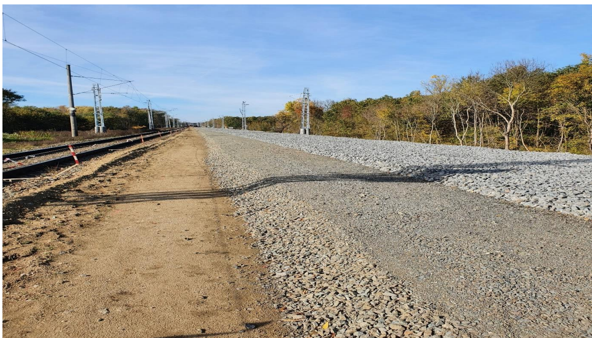
Figure 5. Reconstruction of the railway superstructure (old conditions on the left, new conditions on the right); photo by the author
