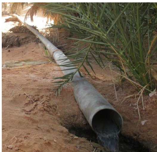
Figure 13. PVC pipes of different diameters occupy the gardens (Photo: Ghachi and Remini, 2013)
