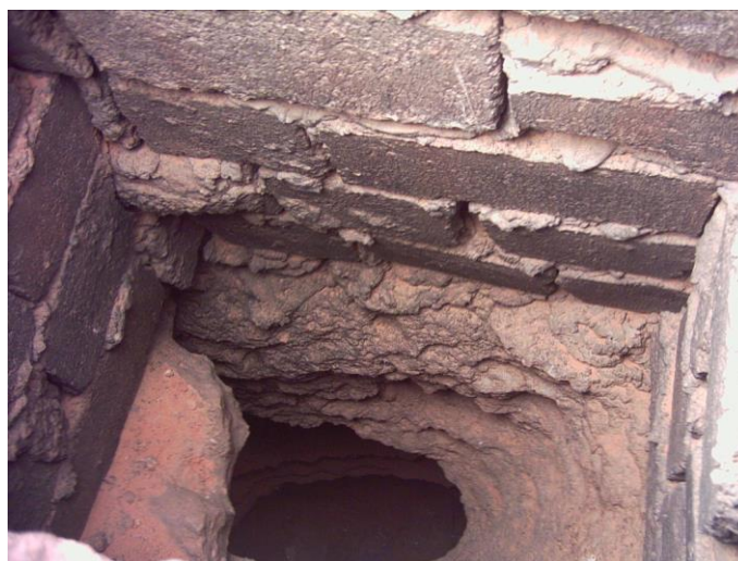
Figure 9. A square cinder block coping in a well ventilation of a Foggara in Timimoun (Photo: Remini, 2008)
