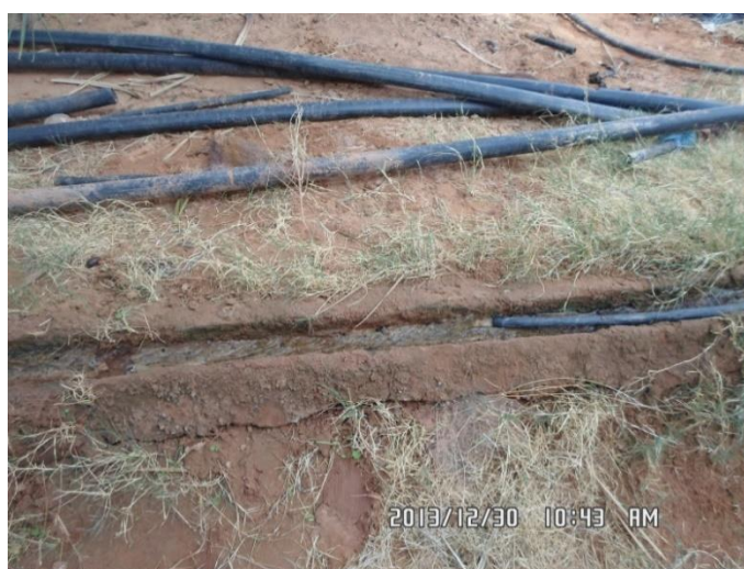
Figure 11. Pipes instead of Souagui in the palm grove of Touat, Gourara and Tidikelt (Photo: Ghachi and Remini, 2013)
