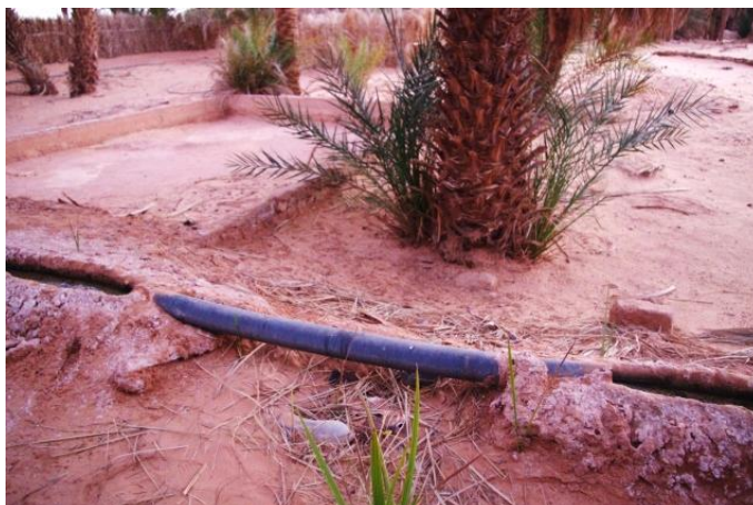
Figure 12. Foggara de Tafza: Replacing the Souagui by HDPE pipes (Photo: Ghachi and Remini, 2013)
