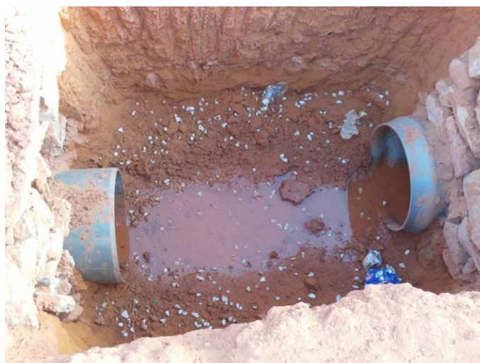
Figure 8. The gallery of the transport part has been replaced by PVC pipes (Photo: Abidi Nouh, 2010)
