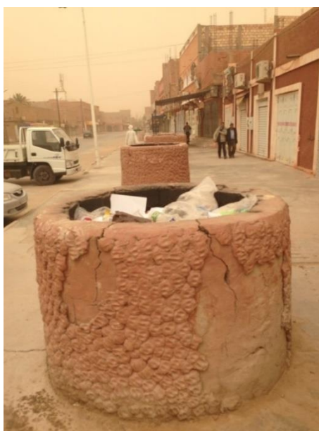
Figure 16. The ventilation shafts used in the towns of Touat, Gourara and Tidikelt regions as public trash cans (Photo: Ghachi and Remini, 2013)
