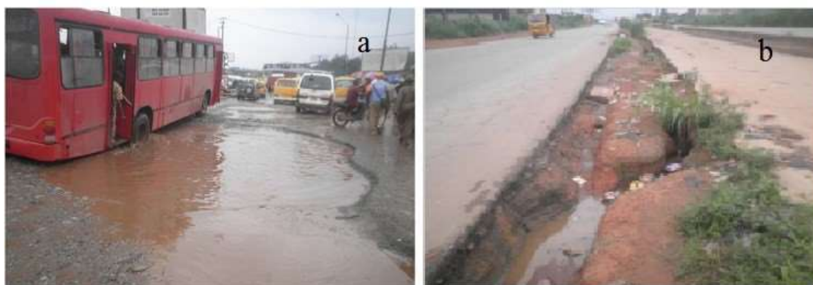
Figure 1. (a) Failed portion of the highway caused by pothole (b) Section of the highway damaged by erosion
