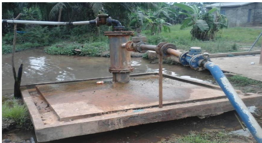
Figure 5. Damaged wellhead equipment [2]
